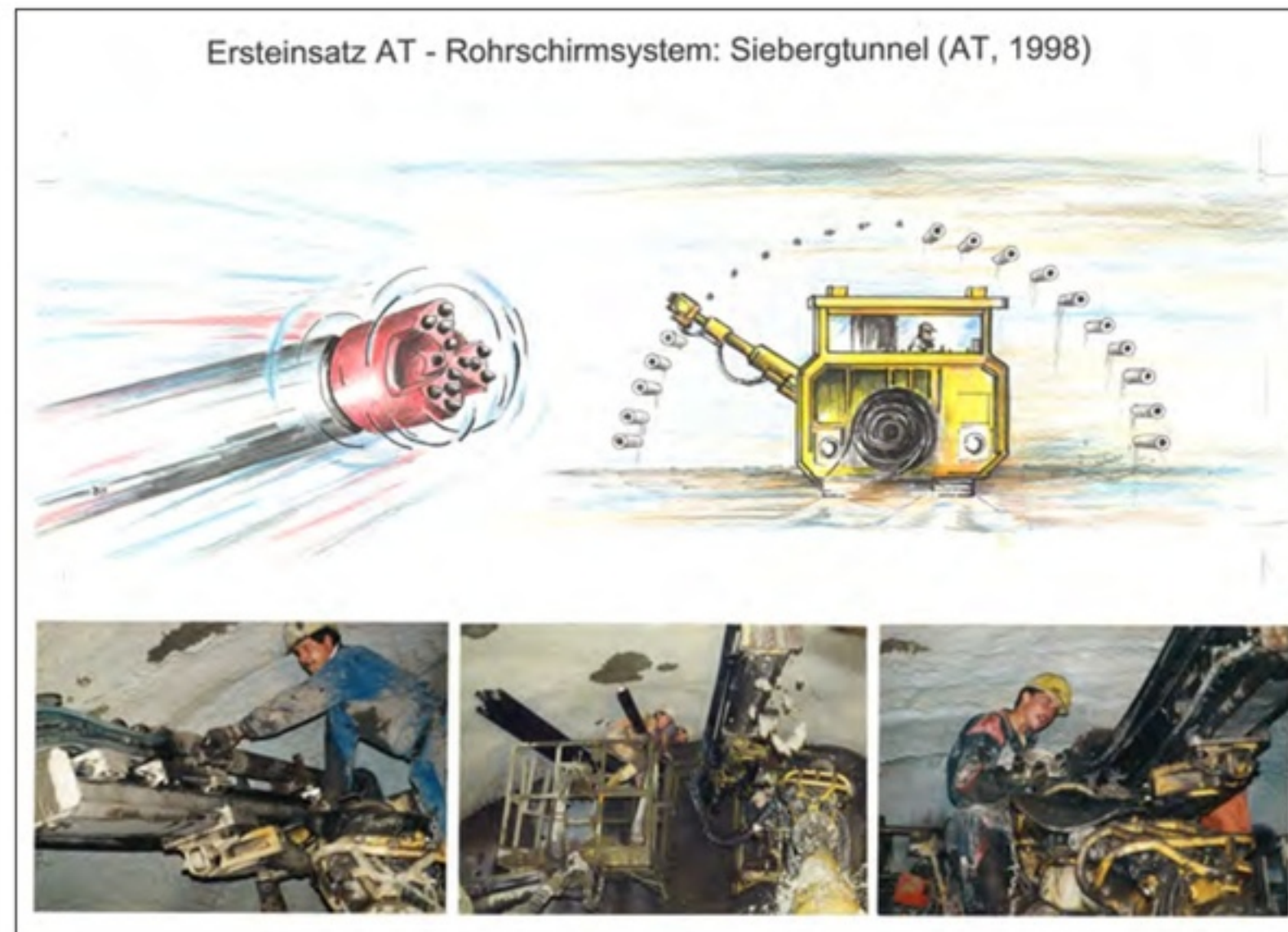
The first ever project to use the AT Pipe Umbrella System was the Sieberg Tunnel in 1998.
