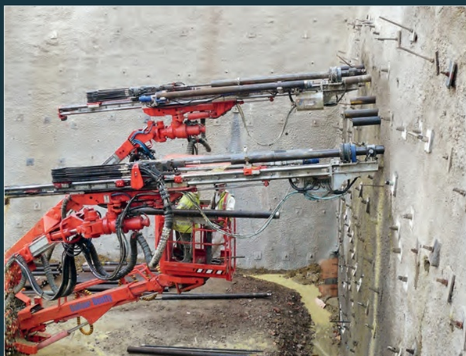
In 2016, the system was used for the tunnel portal for part of the Dulles Corridor Metrorail Project in the US.
